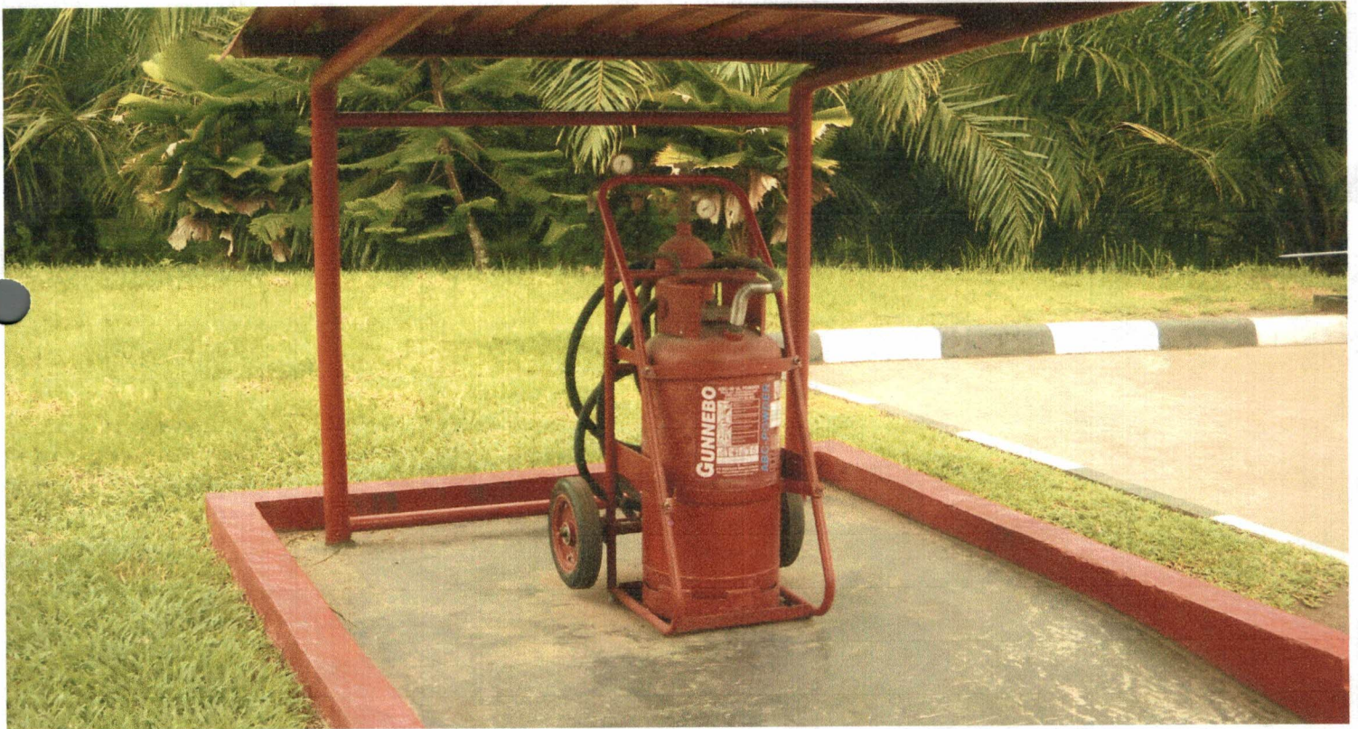
Pompa Racun Api ( Fire Extinguster )
